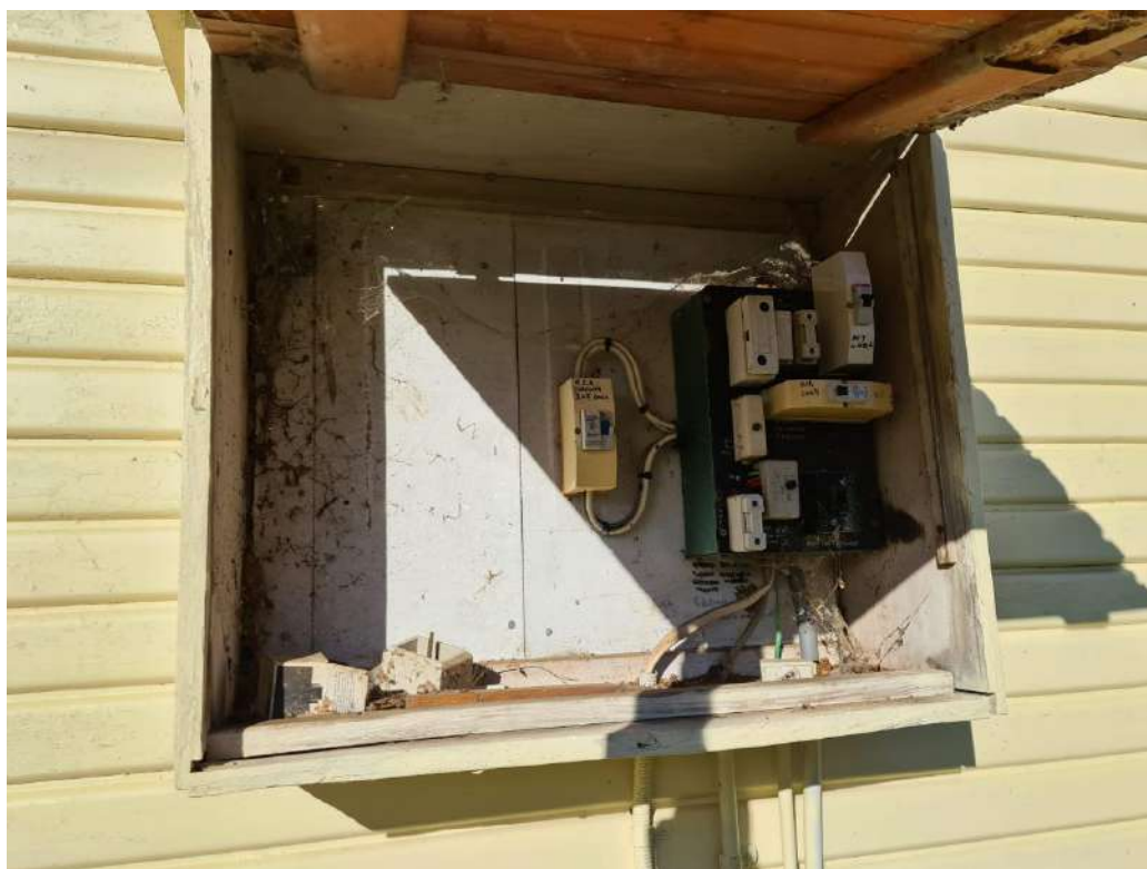
Photograph 2: Fuse Box (Homestead)
