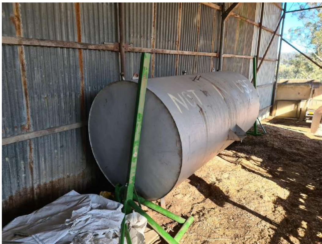
Photograph 14: Another AST tank.
