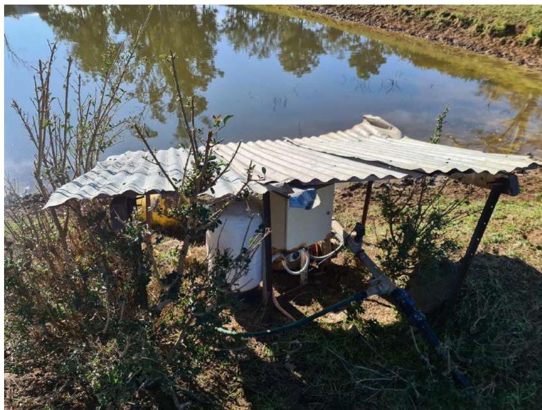
Photograph 20: Dam pump system
