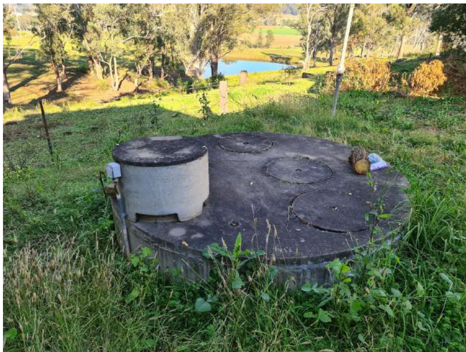
Photograph 5: Septic System. Looking south.
