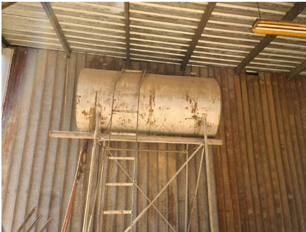
Photograph 13: AST tank with apparent fuel dispenser.
